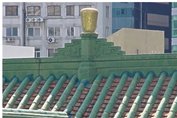
Figure 3: The green and red tiled roof of the church building with its golden "crown" at its apex
